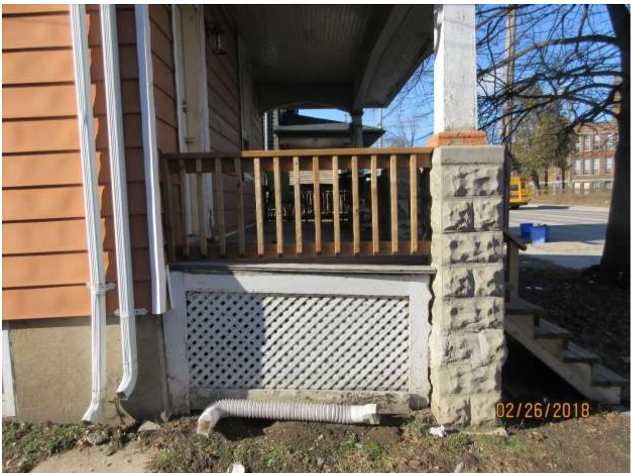
Image 6: Detail of existing south balustrade of the porch of the building at 200 Wharncliffe Road North.
