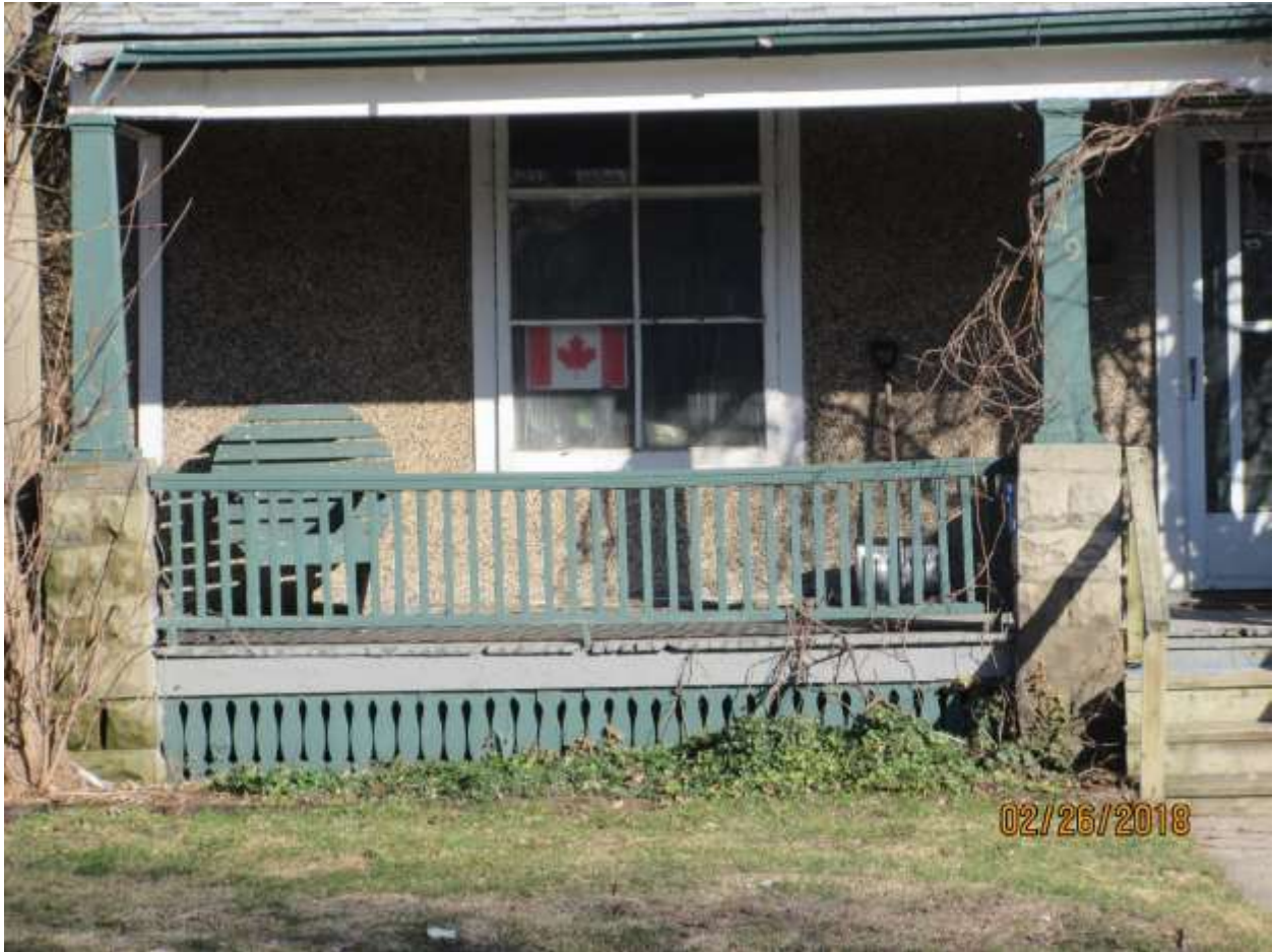
Image 9: Detail of porch balustrade at appropriate height with appropriate details and finish located at the building at 149 Wharncliffe Road North. Note the height of the balustrade is at the appropriate height to match the capstone of the cast concrete plinths.
