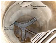
Sanitary sewer manhole with overflow to storm sewer
