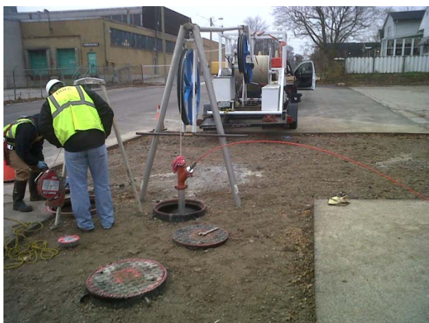
Figure 2 Photo of Pure staff installing the fibre optic cable just south of the intersection of Trevithen and Weston St.
