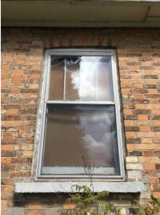
Image 25: Detail view of brick at front elevation showing brick repairs and new window sill
