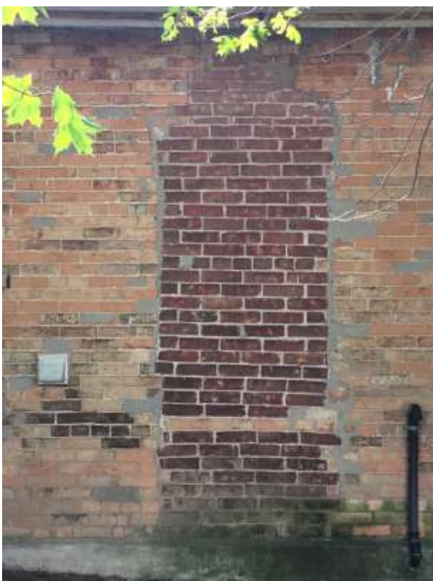
Image 17: Partial north (rear) elevation showing infill brickwork and mortar repairs
