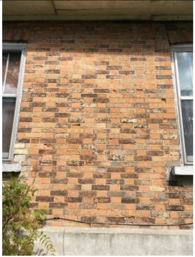
Image 26: Detail view of masonry details at front elevation; parging of exterior foundation wall, drip edge, and Queen closures
