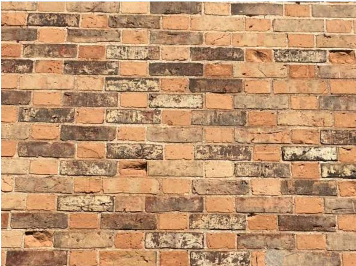
Image 27: Detail view of brick at front elevation; note decorative brick work, Flemish Bond pattern and dichromatic colouring and design
