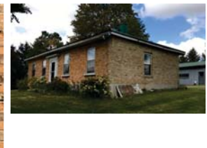
South-east corner view showing new brickwork in differing tone and detailing – full east elevation
