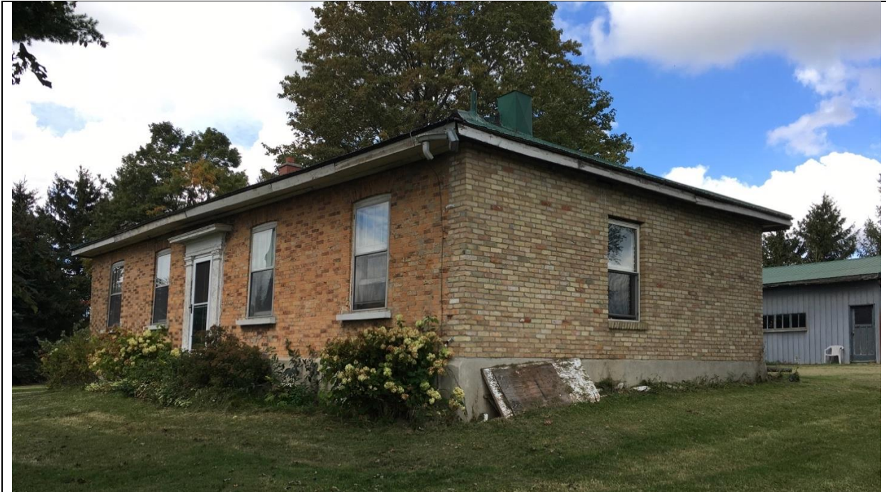
Image 20: South-east corner view showing new brickwork in differing tone and detailing – full east elevation
