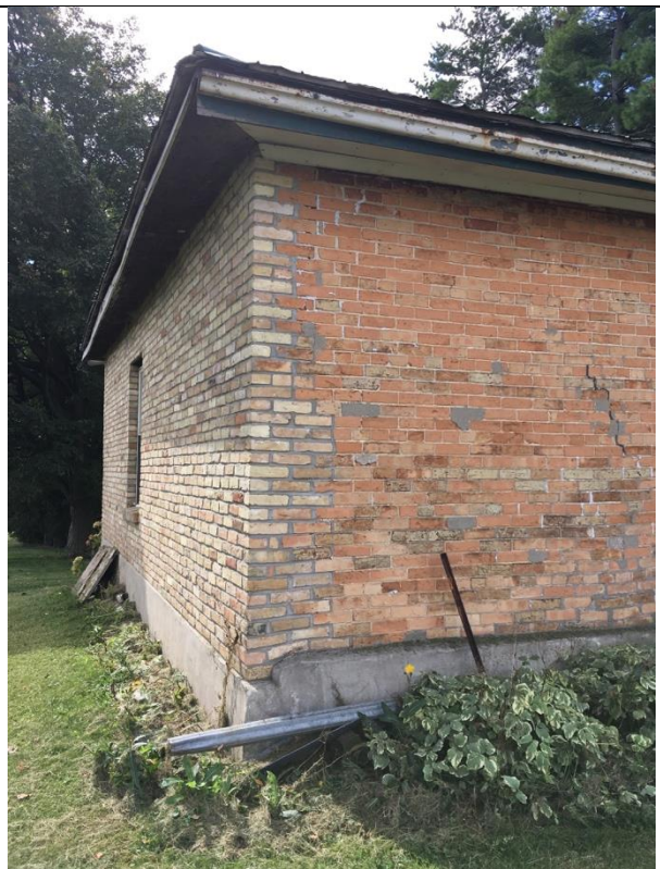
Image 22: North-east corner view showing new brickwork and parging adjacent to original
