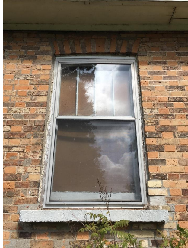
Image 25: Detail view of brick at front elevation showing brick repairs and new window sill
