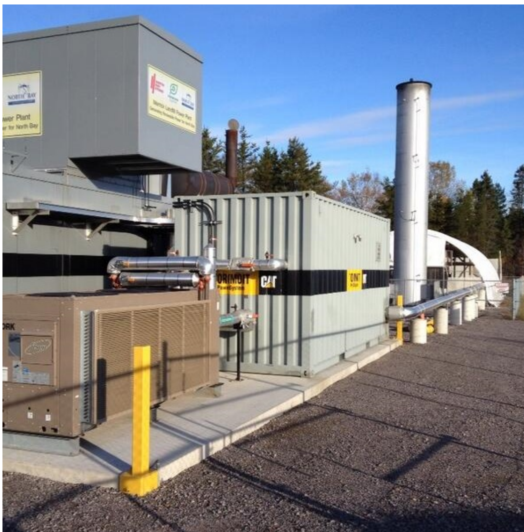
Picture 2 is the 1,600 kW (1.6 MW) landfill gas to electricity facility at the Merrick Landfill, North Bay, Ontario
