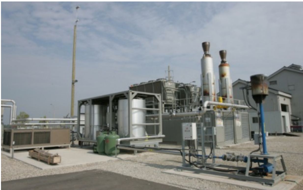
Picture 1 is the 2,100 kW (2.1 MW) landfill gas to electricity facility at the Halton Region Waste Management Site, Milton, Ontario
