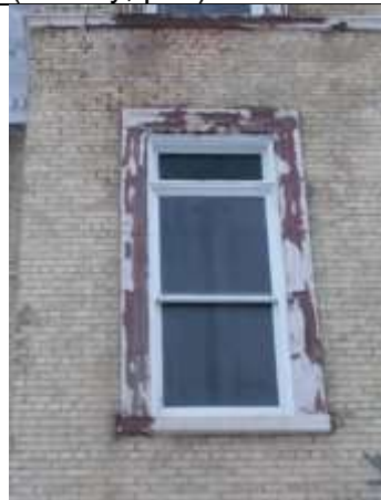
Image 6: Peeling paint revealing underlying sandstone window trim, 2011 (Tausky, p73)
