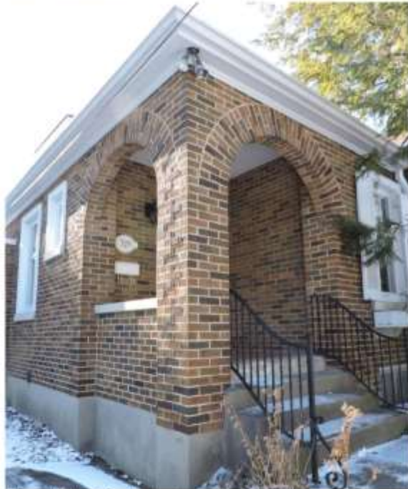
Figure 24: View of the front entrance arches. Also note the overhanging eaves with molded soffit and plain frieze (A. Barnes, 2017).
