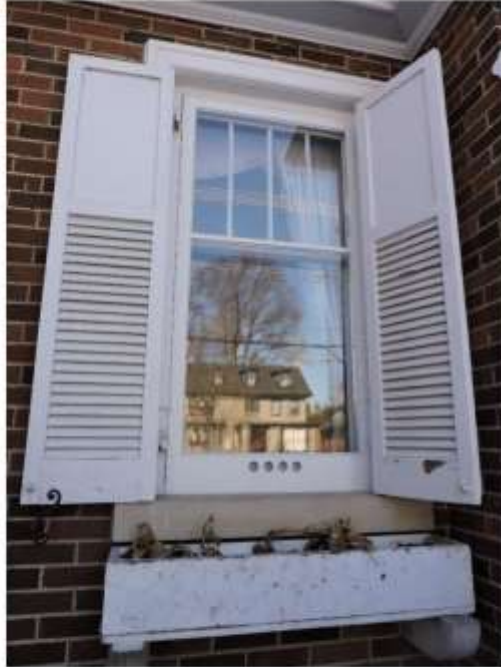
Figure 19: Details of the double hung, 4 over 1, wooden windows and wooden shutters. The storm windows are newer (A. Barnes, 2017).
