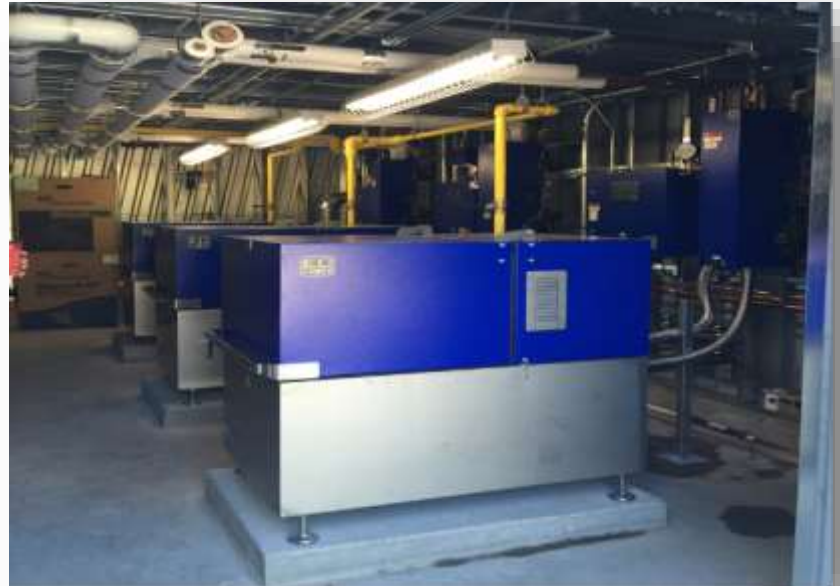
New Combined Heat and Power System
