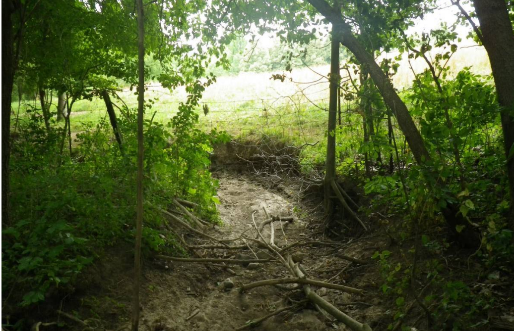
Photo 5 - Reach DCT-1 . Barbed wire and electrical fences near agricultural field boundary mid-reach, with woody debris in channel and basal scour along banks.
