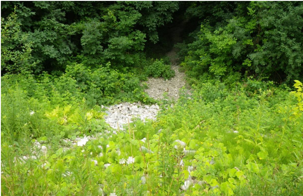
Photo 12 - Reach DCT-3 . SWM pond outlets through 0.4 m CSP, with gravel around outlet.
