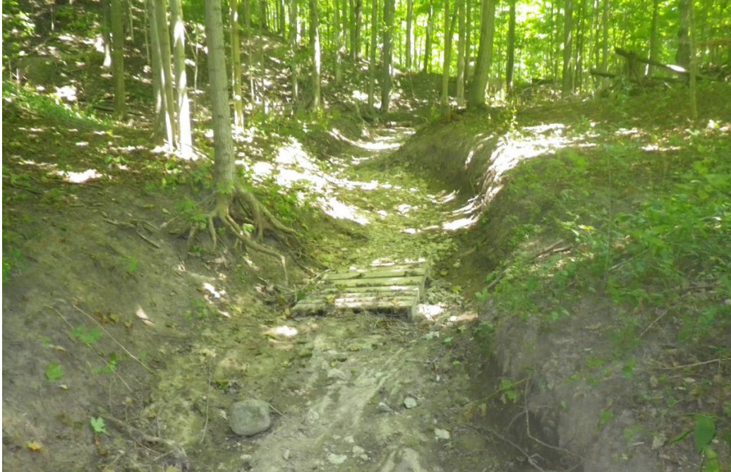
Photo 17 - Reach DCT-4 . Pedestrian bridge located within channel. Reach exhibits low bank heights, exposed tree roots, and basal scour along banks.
