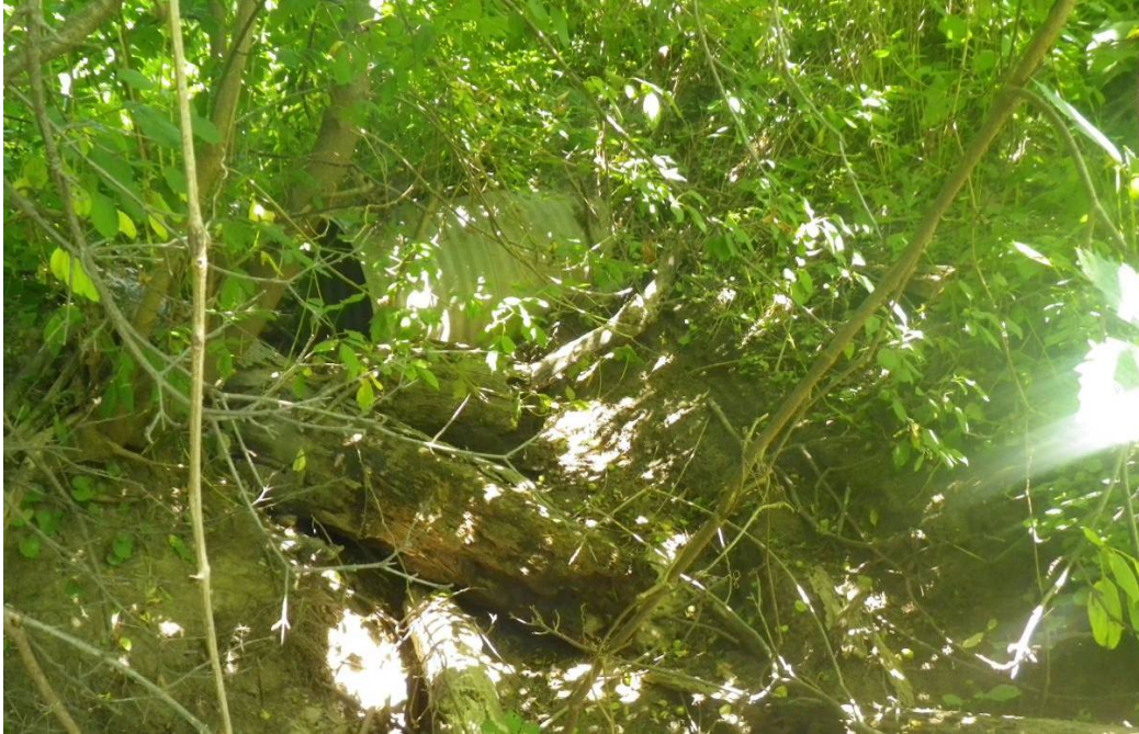
Photo 19 - Reach DCT-4 . Downstream limit crossing Southdale Road West via 1.0 m diameter CSP.
