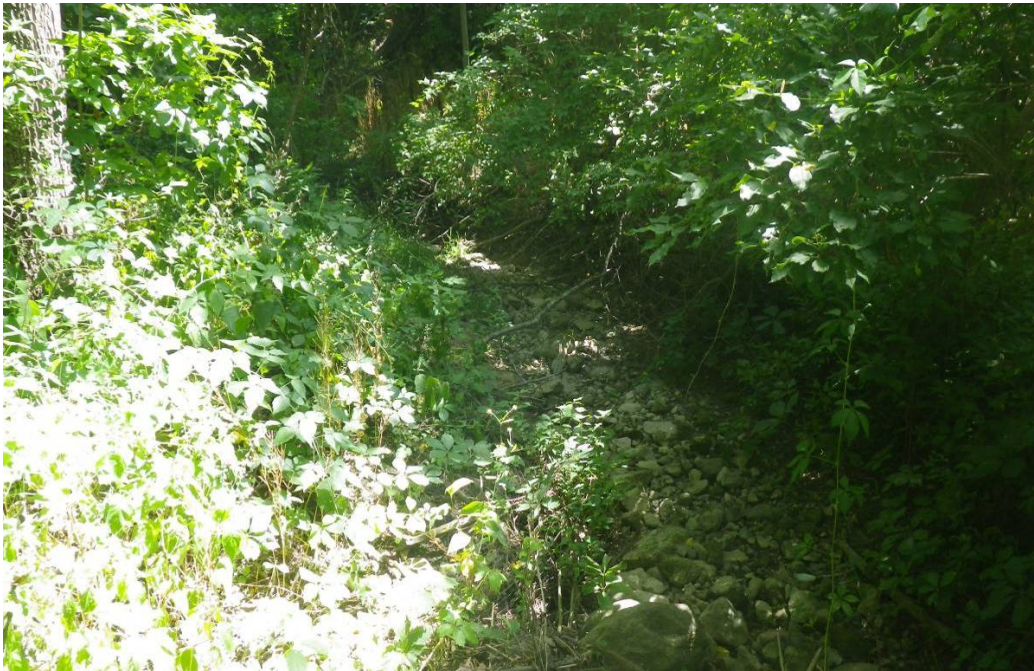
Photo 24 - Reach DCT-5 . Channel becomes defined at downstream end of the reach. Relatively densely vegetated banks exhibit basal scour.
