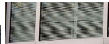
Blinds not always utilized by tenants Photo: FLAP Canada
