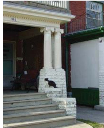
existing porch with original porch detailing (e.g. cast concrete columns, concrete piers)
