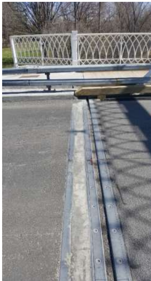
Image 2: Minto East Bridge on April 23, 2017, showing asphalt paving on the left and the "Fiberspan" product on the right at the expansion joint (courtesy Dillon).
