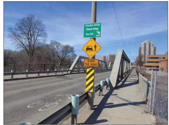
Bridge skew evident in abutments, pier and truss alignments
