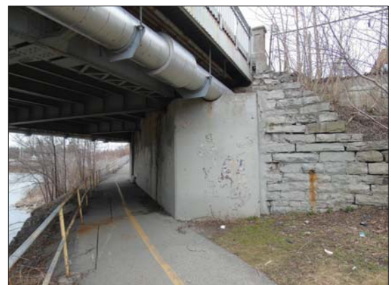
Remnants of decorative stone and concrete end post at north abutment
