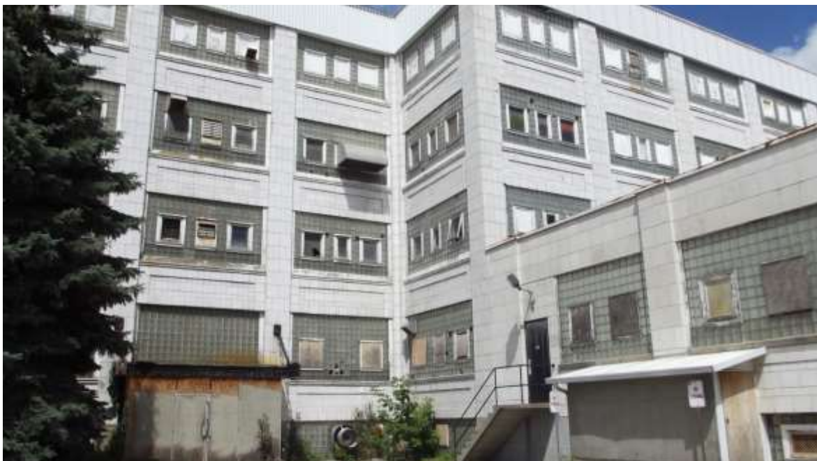
Existing condition of Dundas Street front façade showing east portion of McCormick Factory (both the original four-storey and the post 1950s Candy Store addition to the front of the building – 2015)
