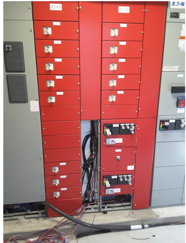
Figure 5b: Construction of a new emergency power MCC in the Low Lift Electrical Room.
