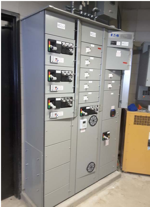
Figure 5a: Installation of a new MCC in the Low Lift Electrical Room.
