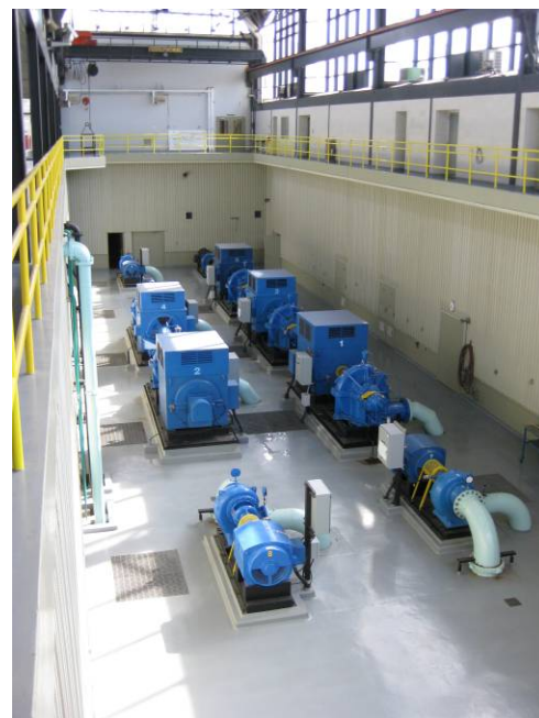
Figure 2: Pumps at the Lake Huron Water Treatment Plant
