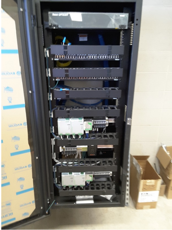
Figure 5c: New networking communications panel, located in the High Lift Electrical Room.
