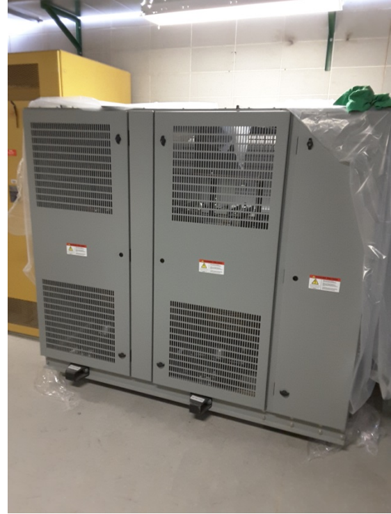
Figure 5d: New transformers in the High Lift Electrical Room, installation pending.
