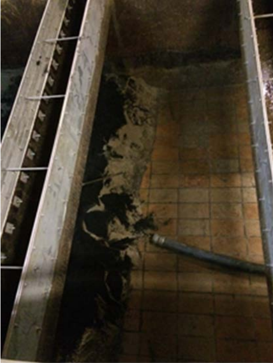
Figure 8a: Removal of the previously existing filter media (sand and anthracite), exposing the old clay tile underdrains.
