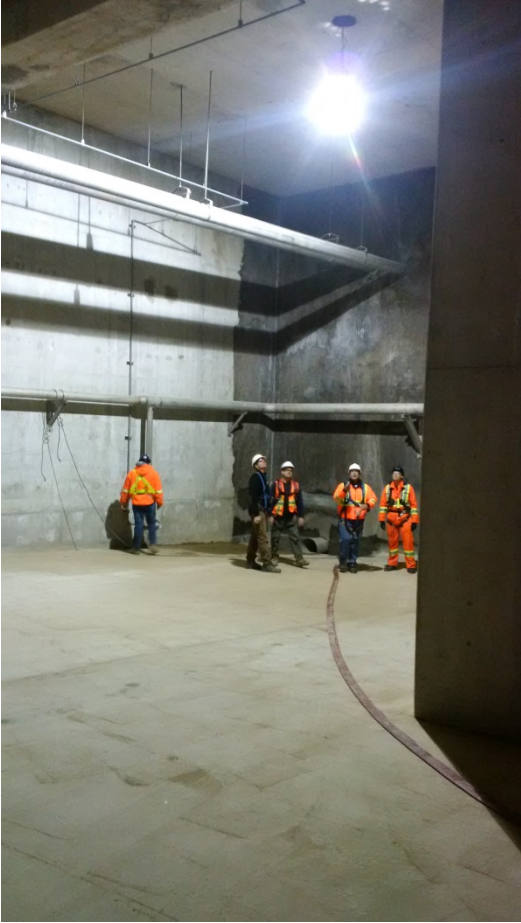
Figure 4a: February 2016 - Inspection of the backwash equalization tank.
