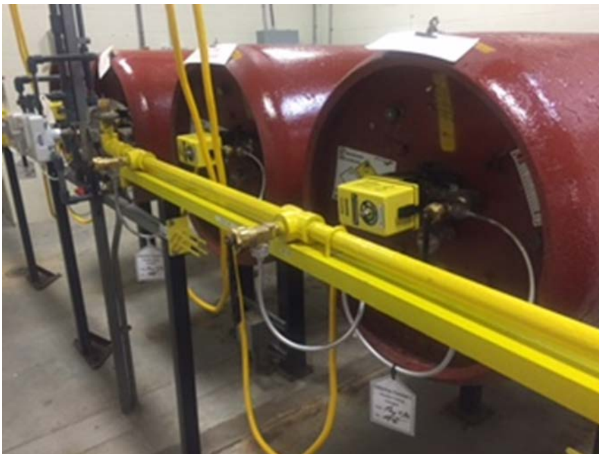
Figure 7: Chlorine tonners with emergency actuated valves
