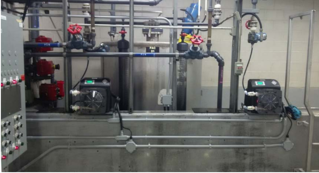
Figure 6: New carbon pumps
