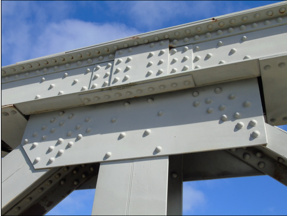
Photograph 12: Riveted gusset plate, part of Warren truss, identified as a Heritage Attribute
