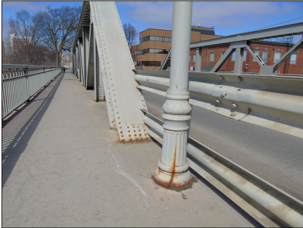
Photograph 14: Decorative base of lamp post located in the middle of the bridge on each side, identified as a Heritage Attribute
