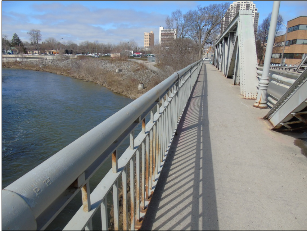
Photograph 16: Railing on west side of the bridge, identified as a Heritage Attribute
