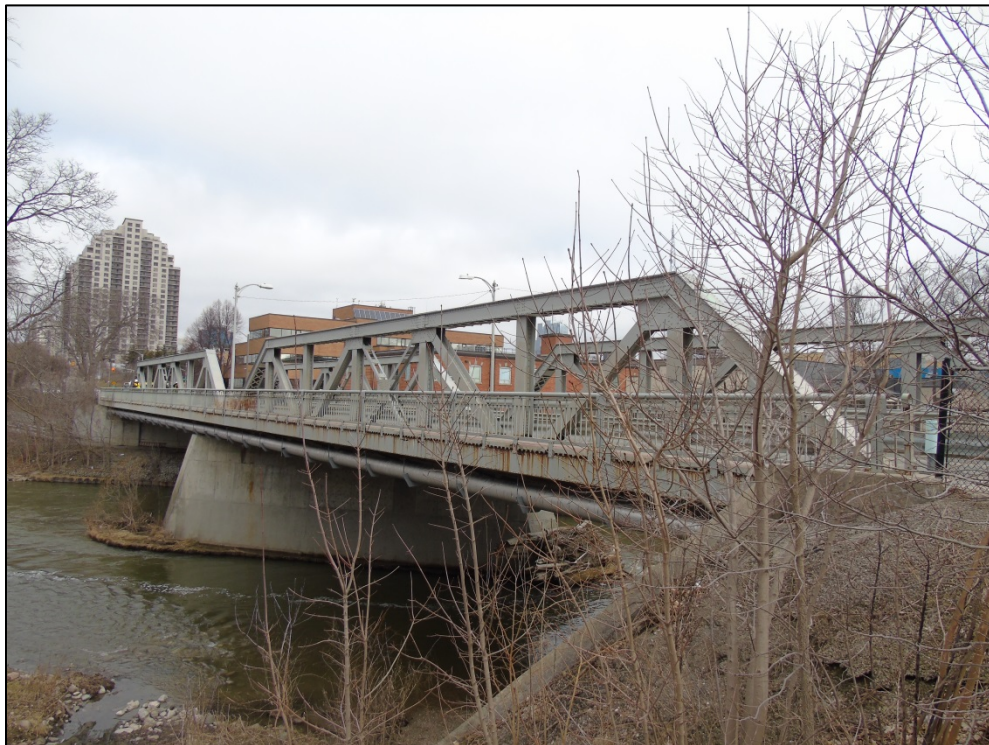
Photograph 15: West truss. The skew of the bridge is not highly visible from photographs; however the skew is identified as a Heritage Attribute. The skew is most visible from aerial imagery or historic mapping.
