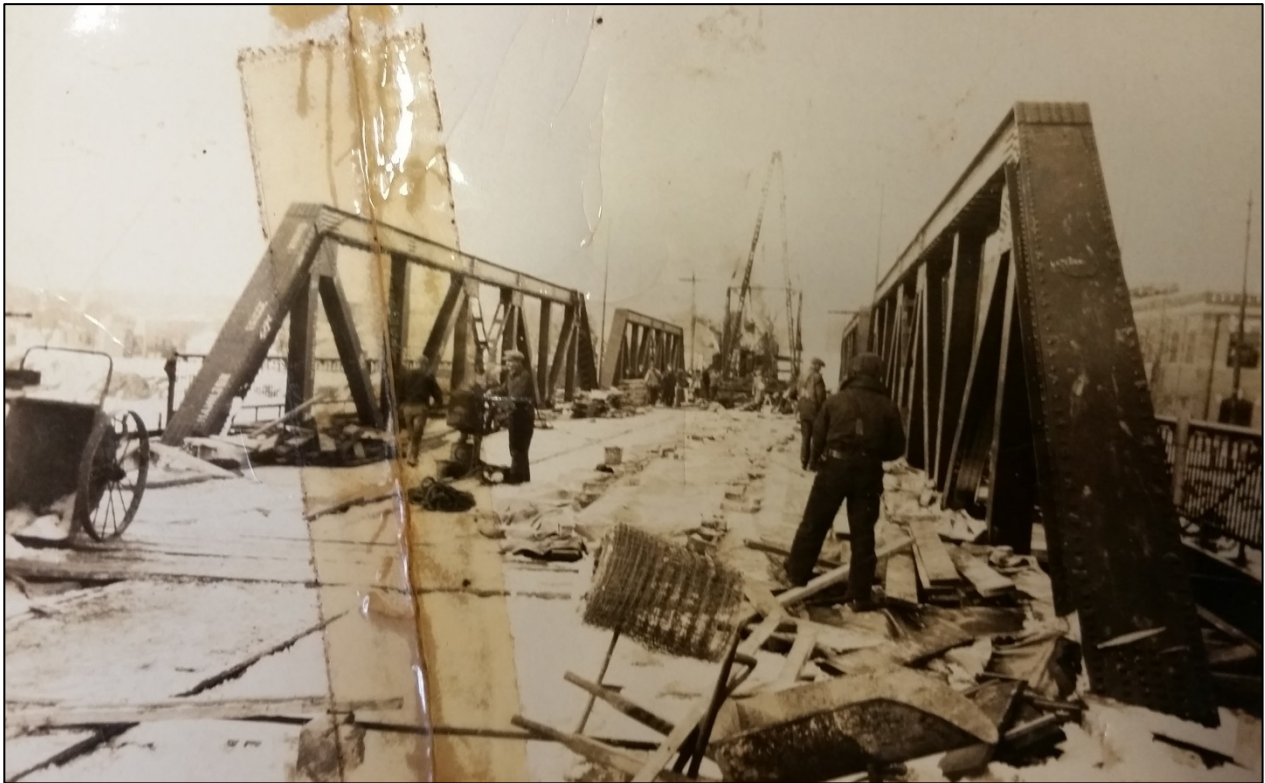
Photograph 5: Victoria Bridge under construction in 1925 showing trusses nearing completion (Victoria Bridge Clippings File, London Room)
