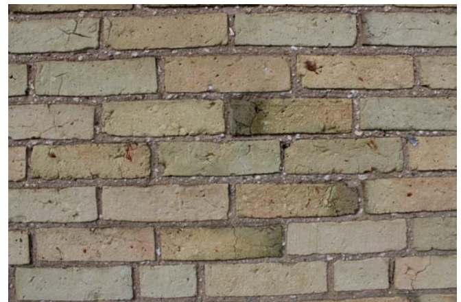
34. Detail of field brickwork. The rough surface and loss of the smooth "skin" may accelerate deterioration.
