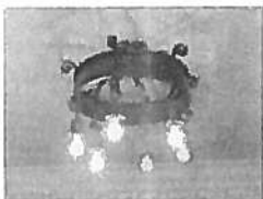
Foyer Ceiling Light
