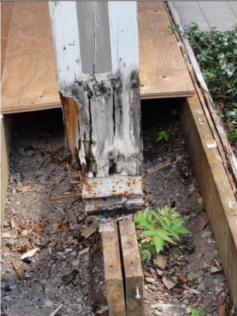
Image 5: Deteriorated column footing
