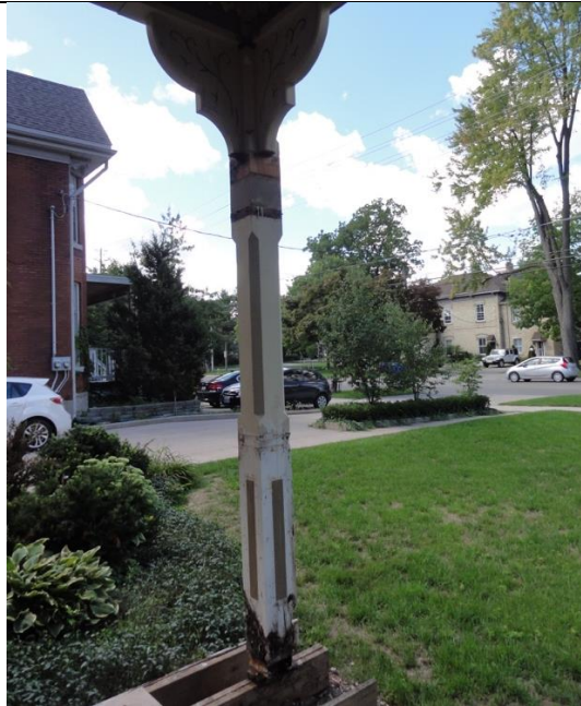
Image 6: Deteriorated column base
