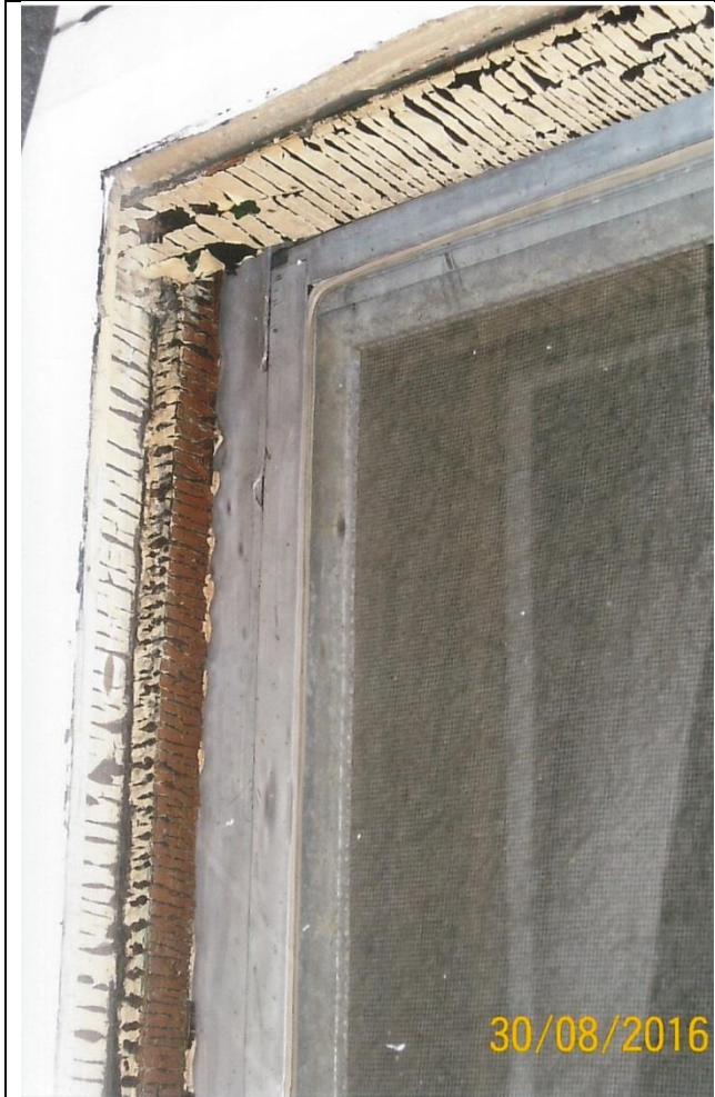
Image 11: Detail of exterior condition of window frames (B. McDougal).
