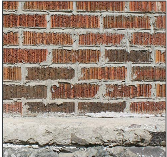
7. Modern Portland mortar repairs are poorly exceeded and virtually impossible to correct.
