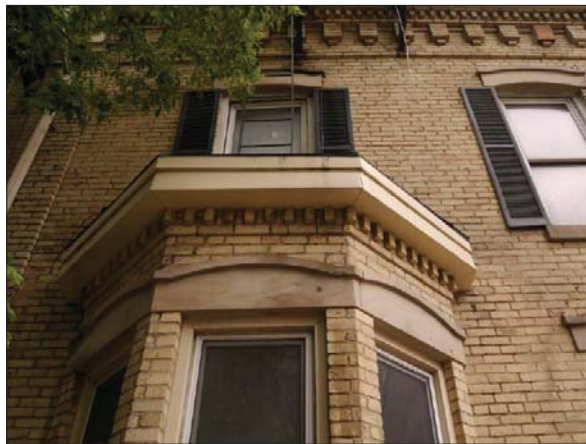
The windows on Camden Terrace are unique because the headers at the top of the windows curve, then level off at the corners. Over the bay windows, they all connect.
