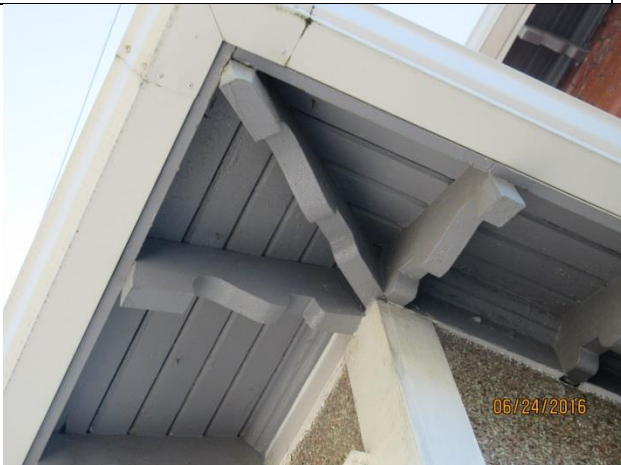
Image 7: Detail of the sculptural projecting verge and sloping tongue and groove soffit on the main roof of the building.
