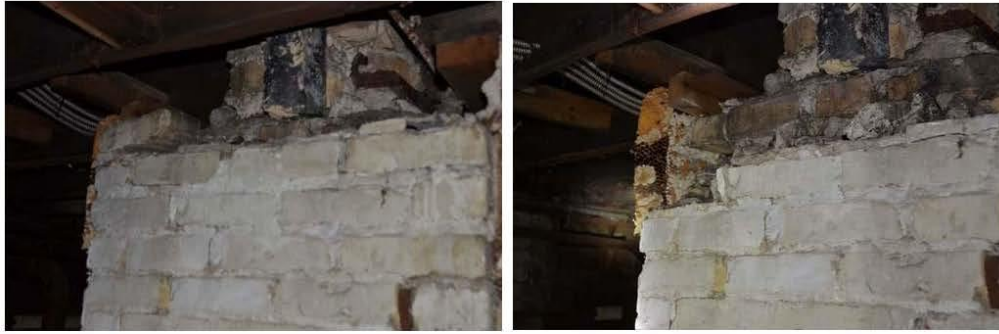
Photo No. 05 & 06: Crumbling Masonry Pier
