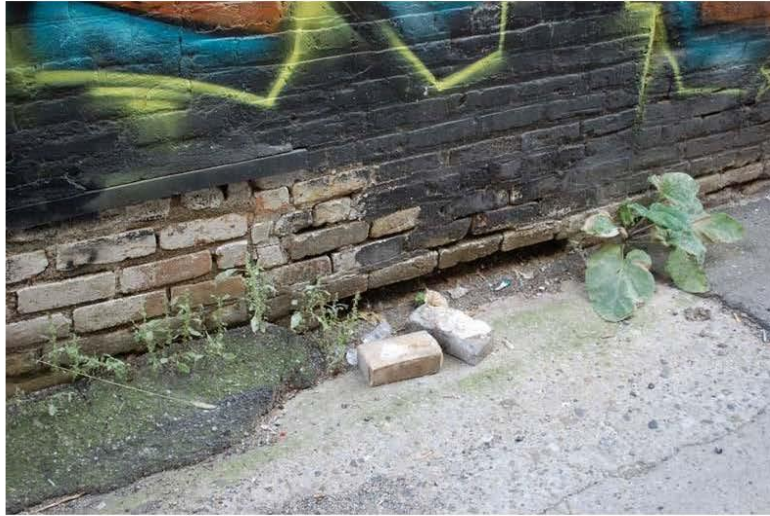
Photograph 14: Missing brick units and missing mortar at grade.
