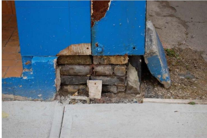
Photograph 5: Brick deterioration at the base of pier on the north elevation. Loss of mortar.
