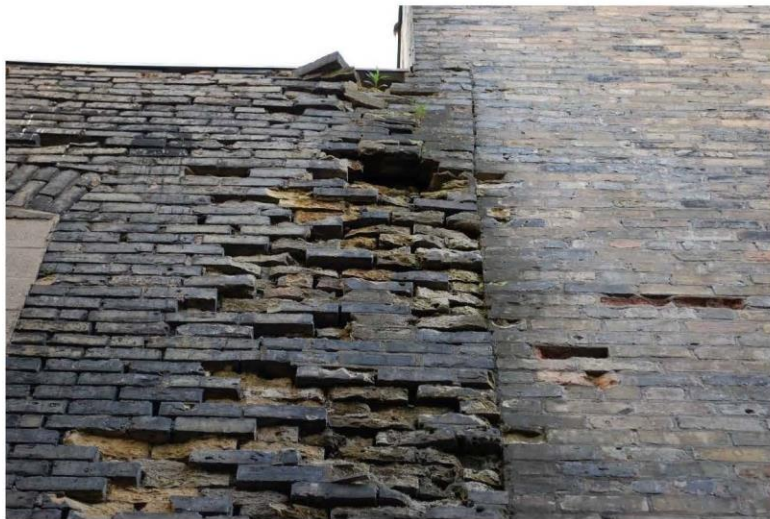
Photograph 19: Masonry at the joint between the two and three storey sections was in extremely poor condition. Note the bricks 'ready to fall' near the top of the wall, plus missing and shifting bricks were observed.
