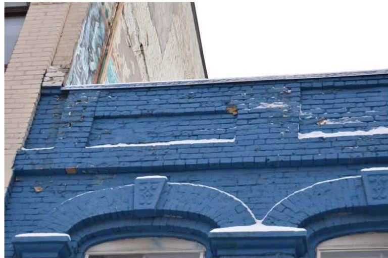
Photo No. 02: Delaminating Masonry Parapet
