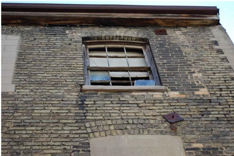
Photograph 26: Broken window at the third floor of the south end of the west wall.
