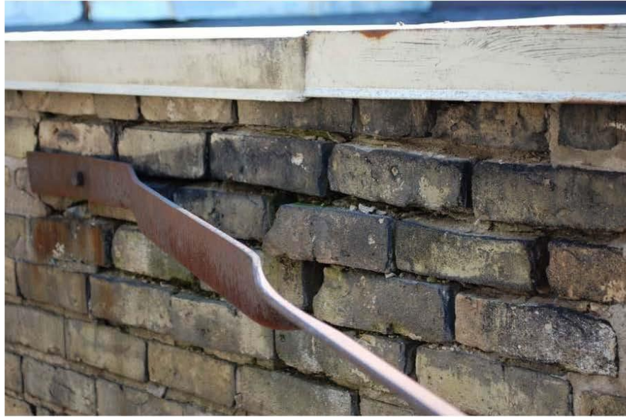
Photograph 12: Parapet deterioration at the anchor for the fire escape.
