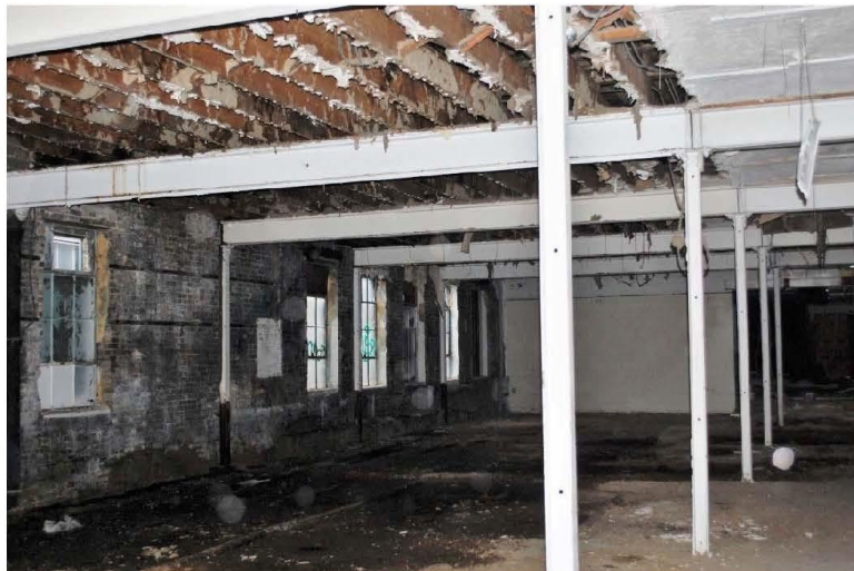
Photograph 44: Approximately 1" +/- movement of sheathing away from wall. No positive connection between roof framing and masonry.
