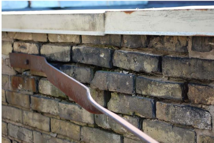
Photograph 21: Parapet deterioration at the anchor for the fire escape.
