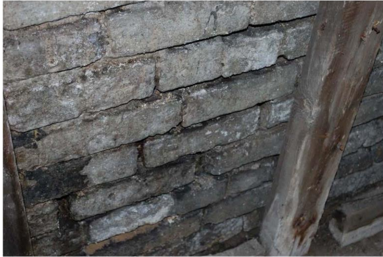
Photograph 6: Basement foundation wall with missing mortar. This type of deterioration was observed in all foundation walls in selected areas.
