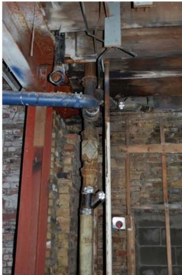
Photograph 50: Water staining of second floor joists due to roof leaks.
