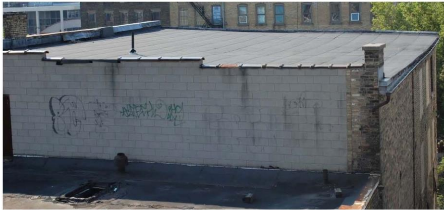
Photograph 33: North wall of south addition. Hollow concrete block capped with clay tile capping.
