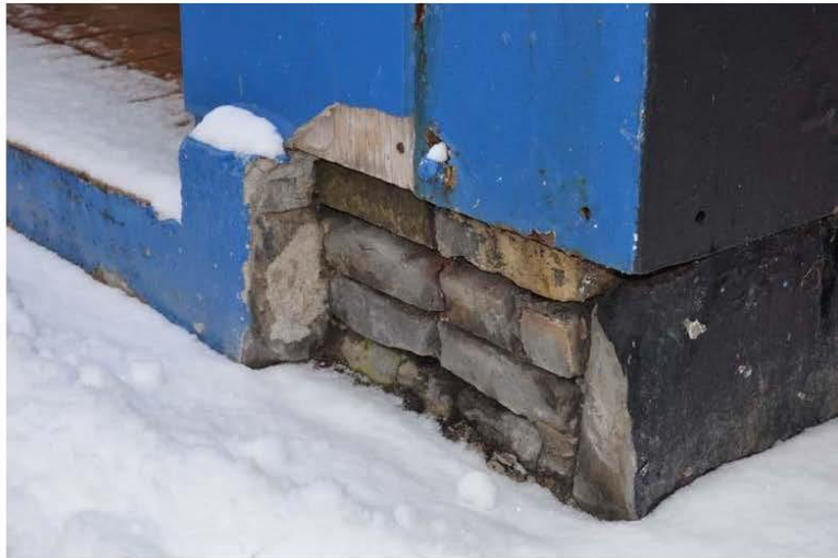
Photo No. 10: Deteriorating Foundation Wall
