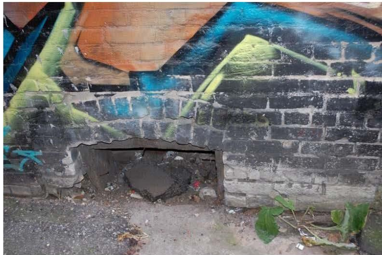
Photograph 13: Mortar deterioration and missing brick units at grade.
