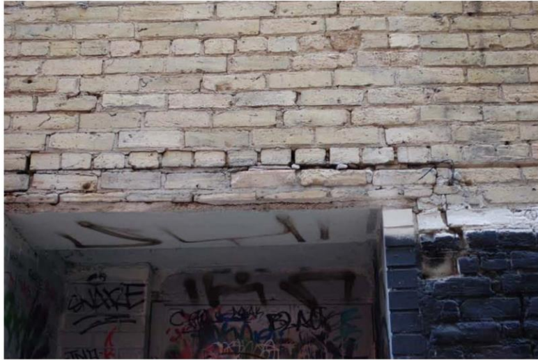
Photograph 9: Mortar loss above the doorway lintel on the west elevation.
