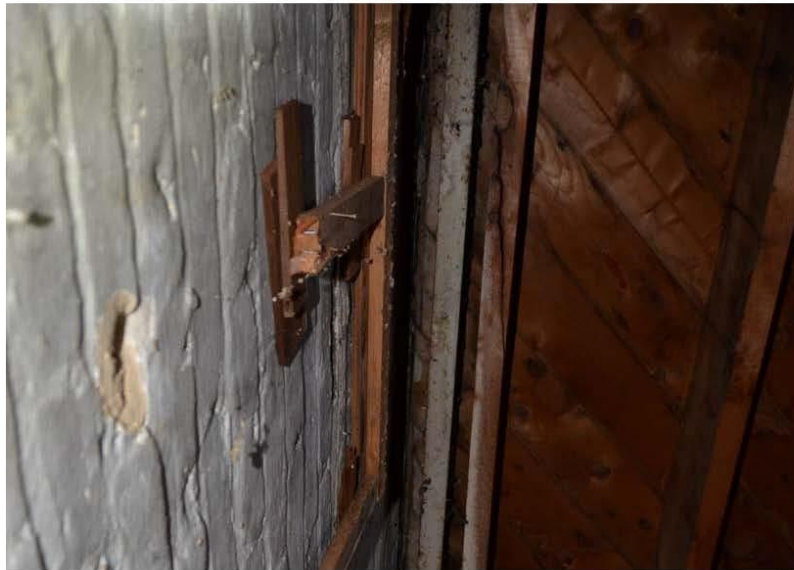
Photo No. 04: Floor Diaphragm Separated from Shear Wall
