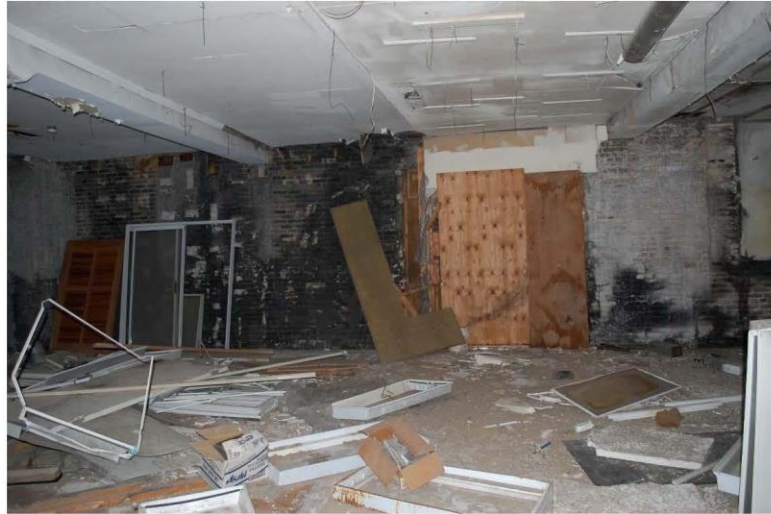
Photograph 39: Interior of the south wall at the second floor level. Note the two bulkheads concealing timber beams. Timber joists span in the east-west direction.
