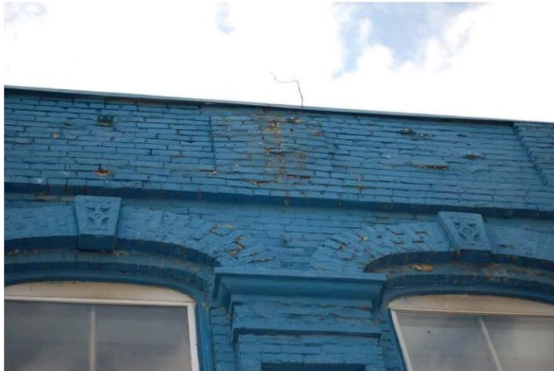
Photograph 6: North elevation near the middle of the wall. Outward brick movement and mortar deterioration at the parapet level.
