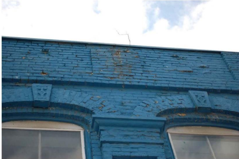
Photograph 15: North elevation near the middle of the wall. Outward brick movement and mortar deterioration at the parapet level. 'Tree' growing out of masonry indicating the presence of growing medium and ample water.
