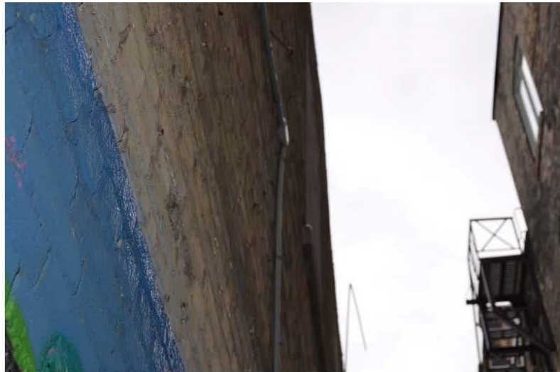
Photo No. 09: Bow out in West Wall
