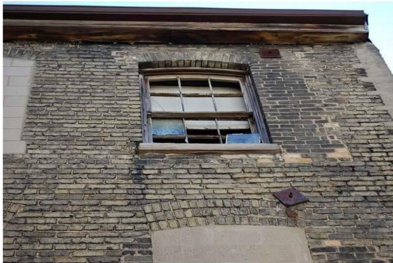
Photograph 19: Broken window at the third floor of the south end of the west wall.
