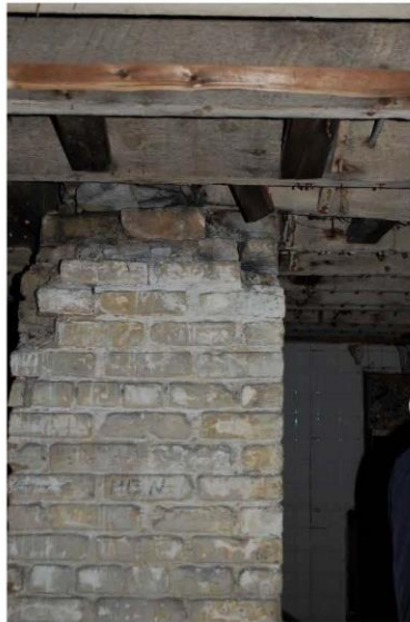
Photograph 11: Masonry piers with deteriorated mortar at the top of pier.
