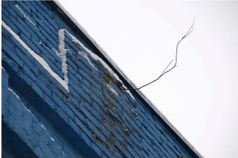
Photo No. 01: Masonry Parapet with Rooted Sapling
