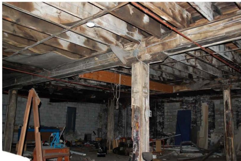
Photograph 38: Timber beams and columns at upper roof level, south addition. Note the tie rods.
