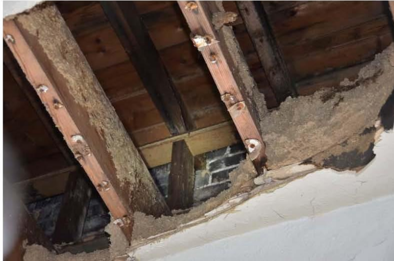
Photo No. 03: Ceiling/Roof Joists at North Parapet
