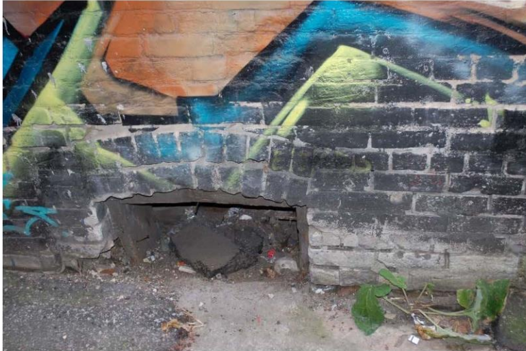
Photograph 22: Mortar deterioration and missing brick units at grade.
