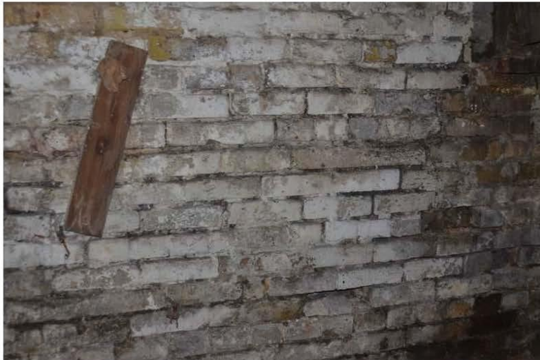
Photo No. 07: Basement Wall with Severe loss of Mortar
