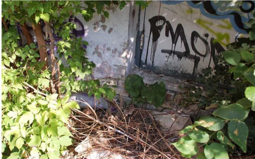
Photograph 8: Foundation wall at south elevation. Plant root and water deterioration of the mortar joints and brick units.
