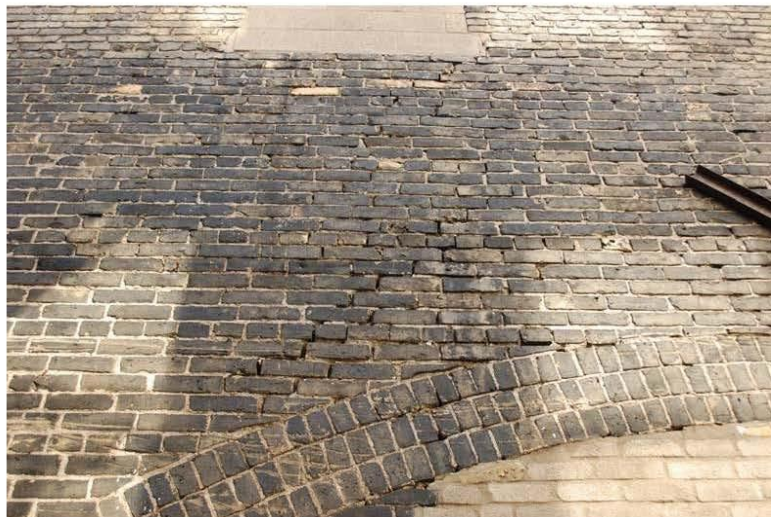
Photograph 8: Blocked-in window openings, mortar deterioration and severe cracking in the west elevation.
