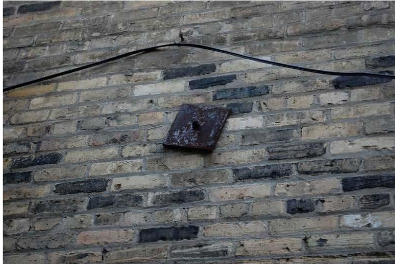
Photograph 16: Tie-back plates on the exterior of the middle addition to connect the floor and wall system.
