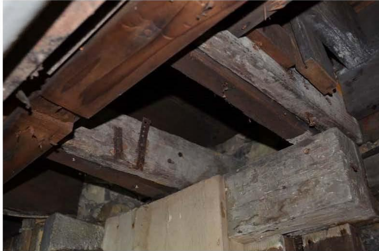
Photo No. 08: Deteriorated Wood Joists
