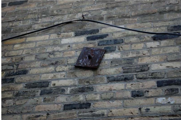
Photograph 24: Tie-back plates on the exterior of the middle addition to connect the floor and wall system.
