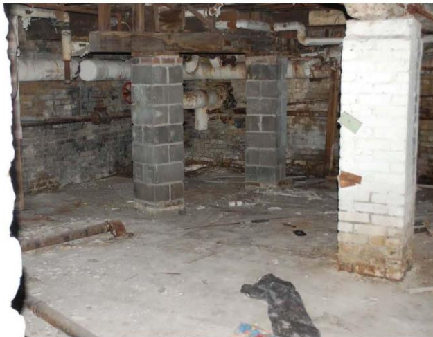
Photograph 9: Partial basement with mortar deterioration in exterior walls and masonry piers (both block and brick masonry).
