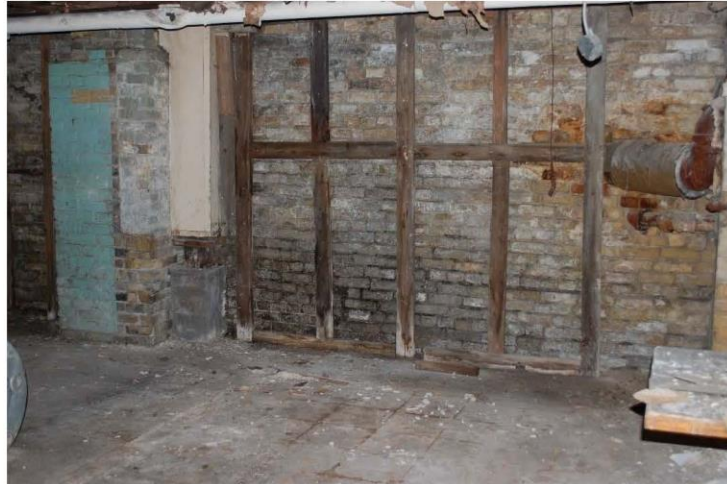
Photograph 10: Deterioration of the mortar joints in the west basement walls was more pronounced at the base of the wall.
