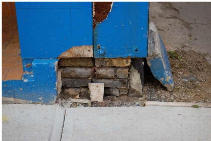
Photograph 5: Brick deterioration at the base of pier on the north elevation. Loss of mortar.
