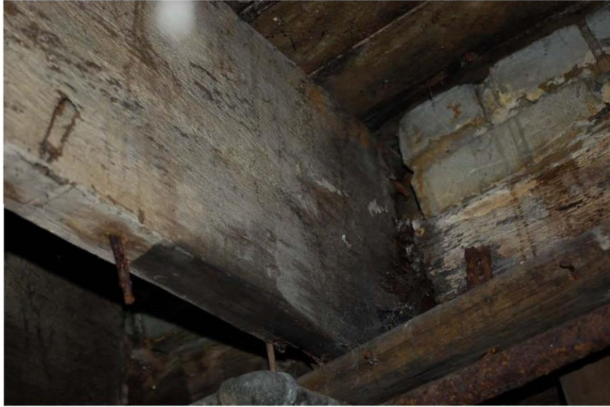
Photograph 52: Water staining and dry rot in main floor joists at the west wall.
