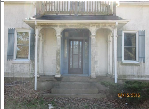
Image 5: Detail of the front entry to the house located at 5067 Cook Road.
