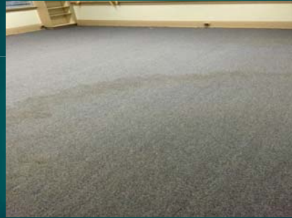
Water Stain – Hidden Mould
