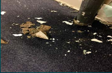
1925 Water Damage and Hidden Mould
