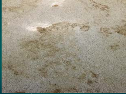
Mould coming through asbestos floor
