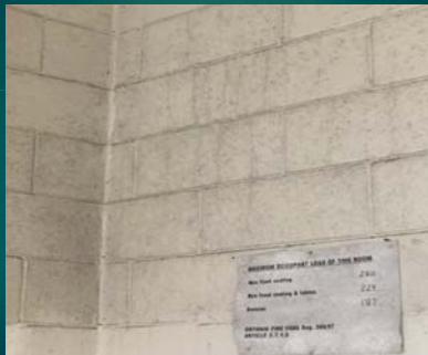
Black Mould in Gymnasium Wall
