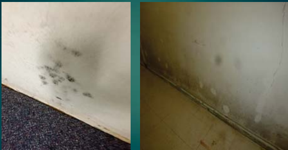
1925 Black Mould on Walls
