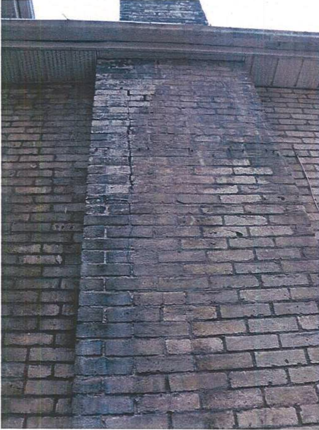
Crack in the brick of the chimney, and deterioration of the mortar joints.
