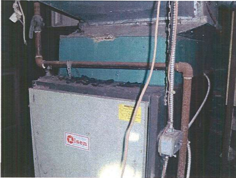
The existing gas furnace heater for building located at 764 Waterloo St.
