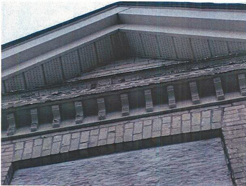
Damage to existing exterior. Metal soffits and fascias are not original.
