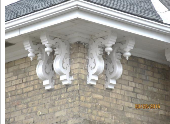
Image 7: Detail of the Italianate brackets on the eaves of the building located at 1656 Hyde Park Road.
