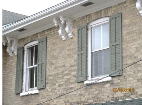
Image 8: Detail of the two-over-two wood windows with aluminum storm windows in front and wooden louvered shutters on the building located at 1656 Hyde Park Road.
