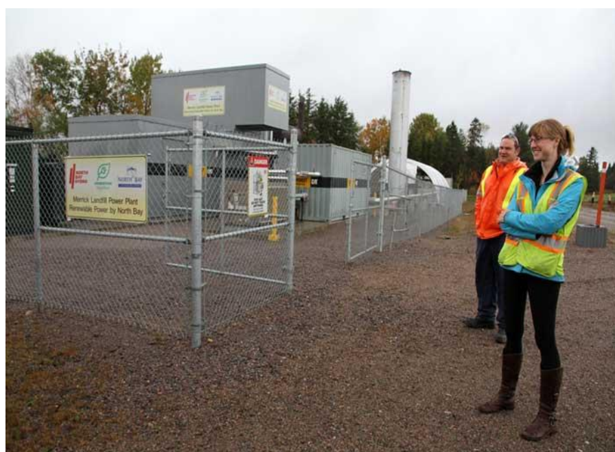
A landfill gas generator (1.6 Megawatt) was installed in 2012 at the Merrick Landfill Site, North Bay, Ontario
