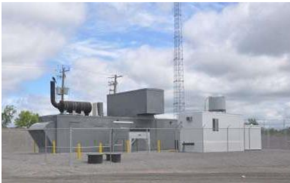
A landfill gas generator (1.6 Megawatt) was installed in 2013 at the Bensfort Road Landfill Site, Peterborough, Ontario
