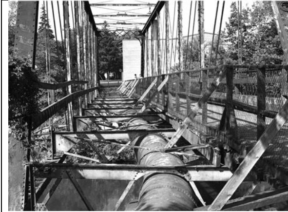
Image 5: Exposed suspender sewer of the King Street Bridge during rehabilitation work (courtesy of the London Free Press , 1958).
