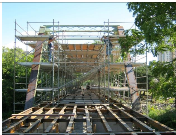
Image 8: Rehabilitation work on the King Street Bridge (courtesy of the City of London, 2010).
