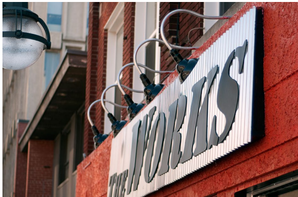
Gooseneck light fixtures used to illuminate signage, Downtown London, ON
