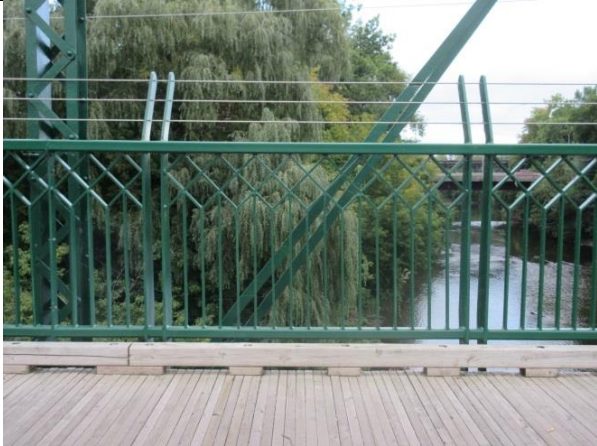
Image 11: Detail of the hand railing, installed as part of the 2010 rehabilitation program (September 29, 2015).
