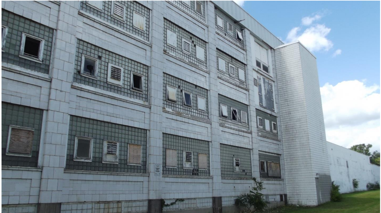
Figure 5 – Existing condition of Ashland Avenue facing façade showing east portion of McCormick Factory (both original 4 storey front portion and 1922-1958 rear addition)
