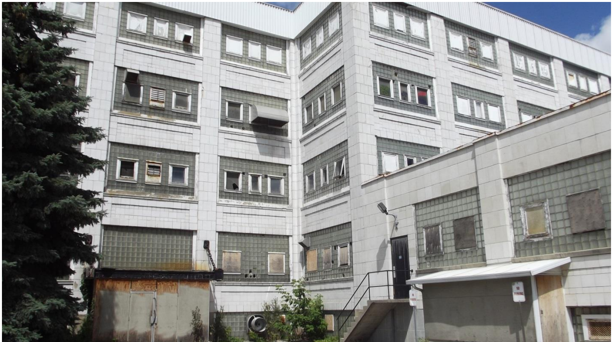
Figure 4 – Existing condition of Dundas Street front façade showing east portion of McCormick Factory (both the original 4 storey and the post 1950s addition to the front of the building)
