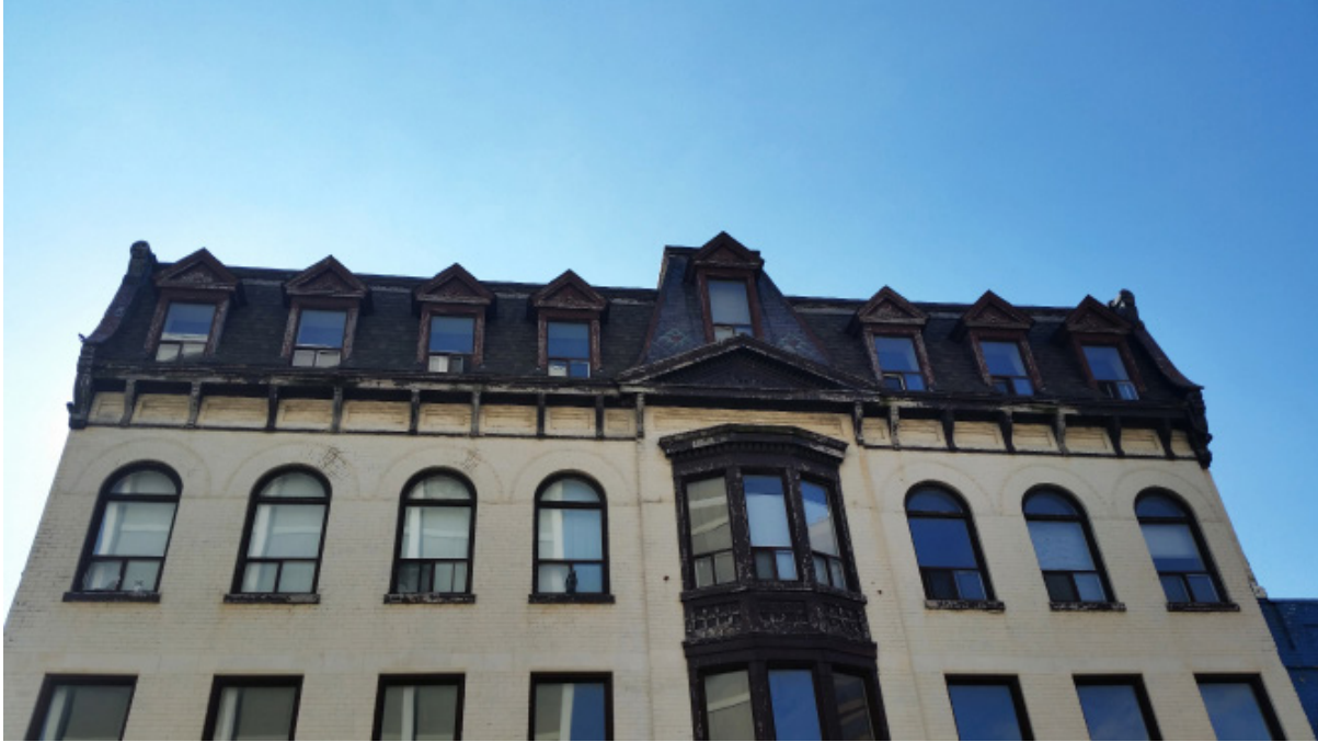
28. 183 King St., arched windows, bay windows, mansard roof and tower (Source: ERA Architects)
