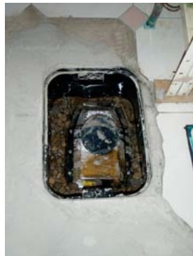
Installed Backflow Valve
