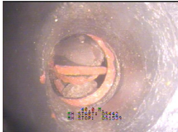
Bruce Street pdc ~ broken
