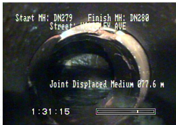
Wolsley Avenue ~ joint displaced
