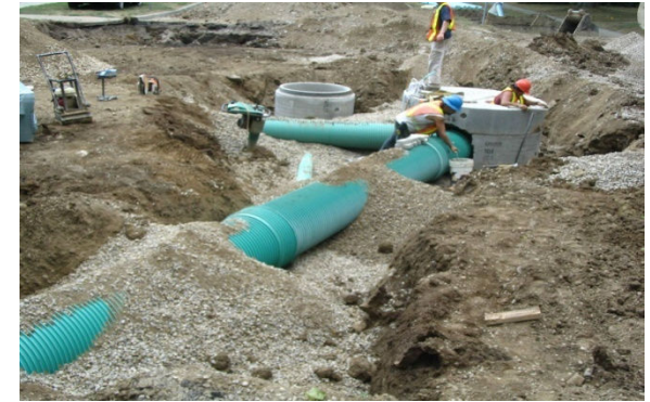
Storm manhole and sewers on Regent St.
