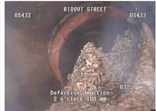
Ridout Street ~ defective junction
