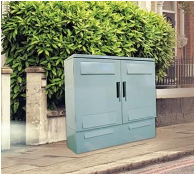
FIGURE 3 – Example of Battery Storage System
