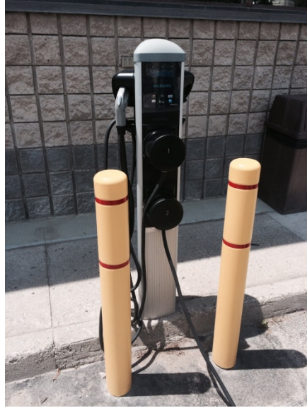
FIGURE 2 – Example of Level 2 Electric Vehicle Charger
