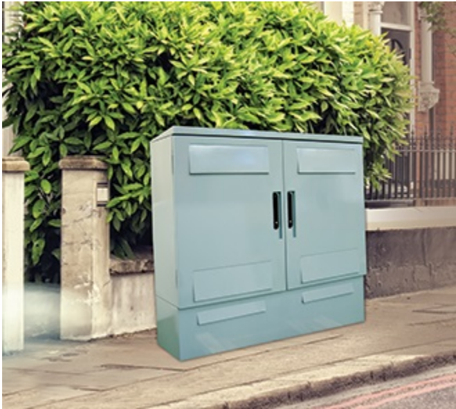
FIGURE 3 – Example of Battery Storage System
