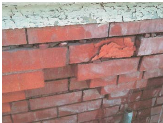
Fig 8: Typical face brick deterioration
