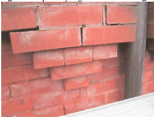
Fig 7: Typical open joints to be repaired
