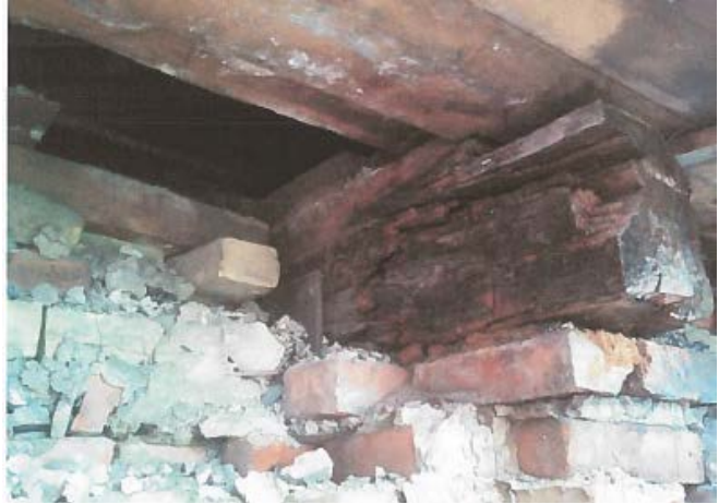
Fig 10: End of wood truss showing deterioration.
