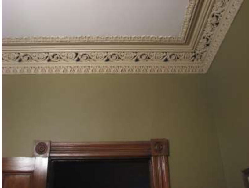
Image 7: Detail of the ornamental plaster work and sample of the wood trim in the double parlour of 77 Price Street (January 28, 2015) (Image courtesy of the property owners).
