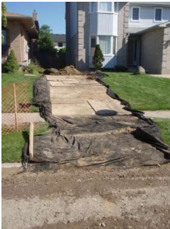
Figure 3: access to receiving pit for installation of storm PDC with lawn protection
