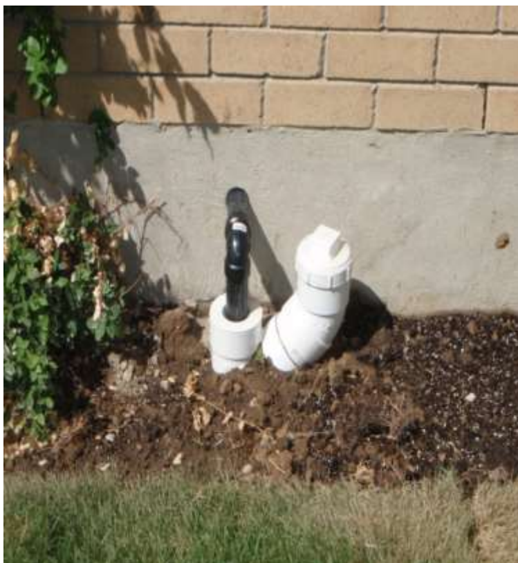
Figure 5: sump pump discharge pipe (black) entering new storm PDC (white)
