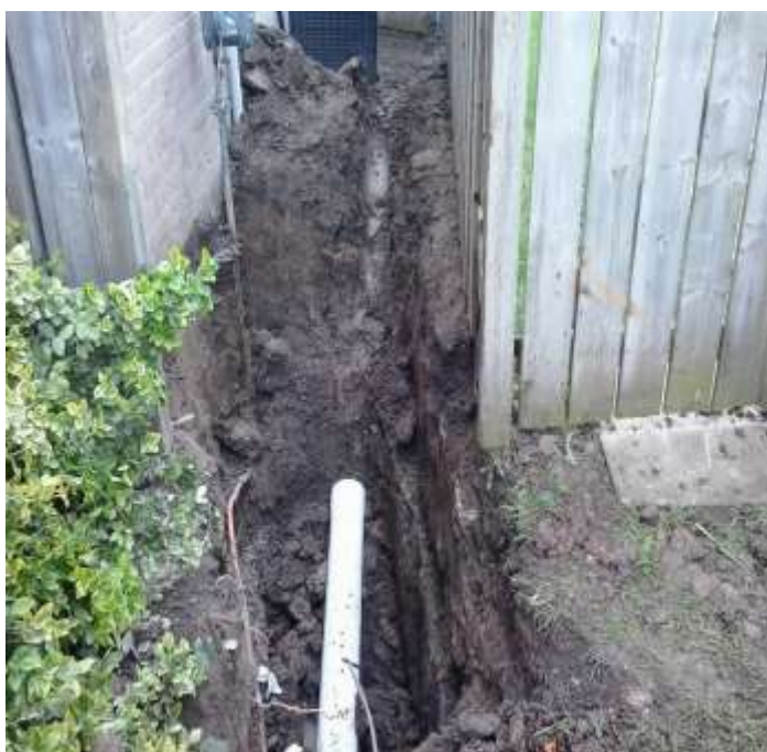
Figure 4: receiving pit to retrieve storm PDC to connect to sump pump discharge pipe
