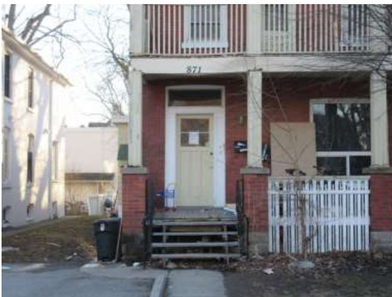
Image 3: Detail of the front steps at 871 Waterloo Street (March 31, 2015).
