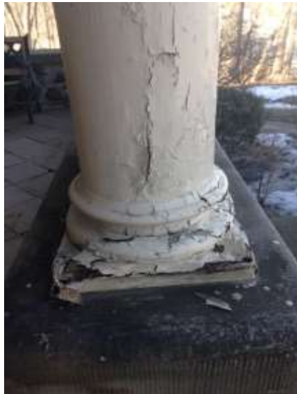
Image 5: Detail of a column at 37 Ridout Street South. Note the existing condition apparent in the photograph (March 2015) (Image courtesy of G. Fonseca).
