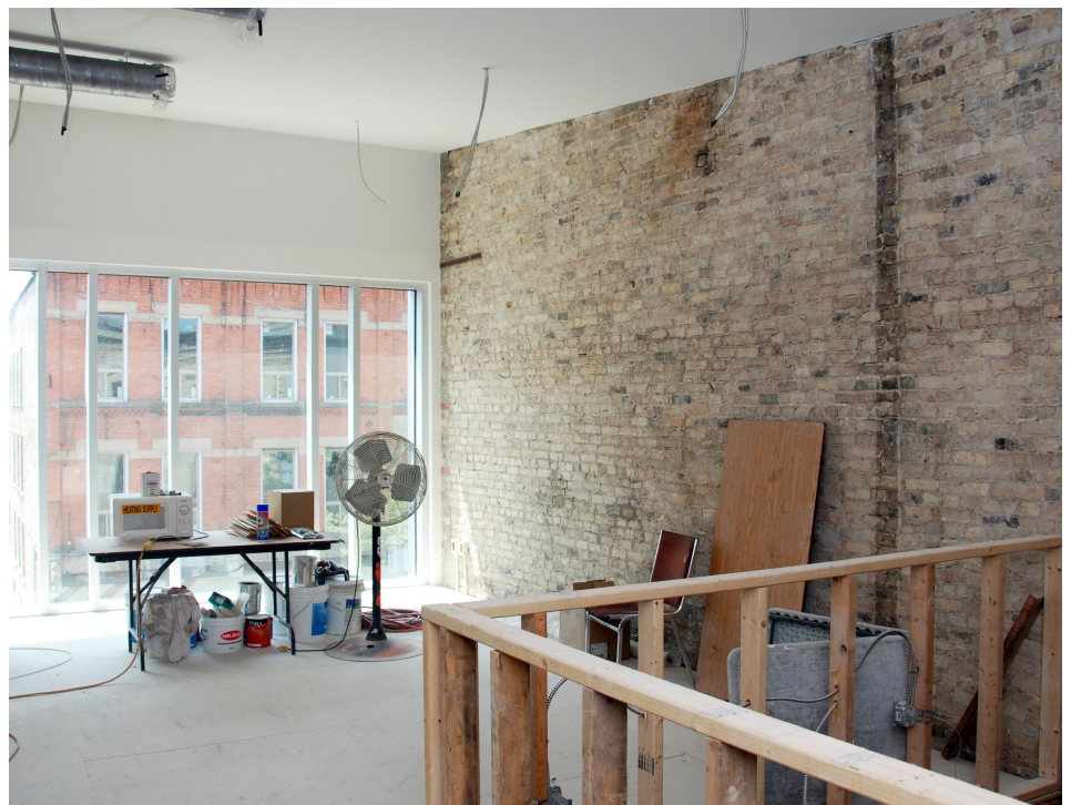
Downtown building renovations in progress and supported through City Loans and grants.
