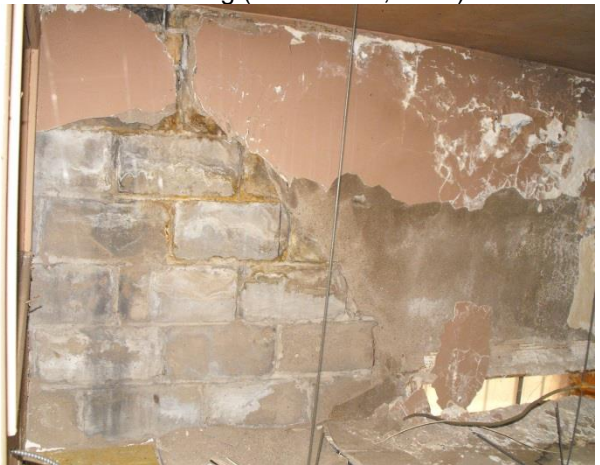
Image 11: Evidence of moisture penetration and settling on the interior (above drop ceiling) (October 24, 2014).
