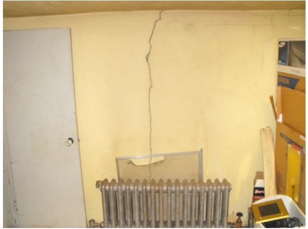
Image 9: Evidence of settling is visible on the interior of the building (October 24, 2014)
