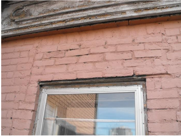
Image 8: Evidence of former repair and structural settling in brickwork (October 24, 2014)
