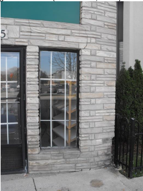
Image 10: Vertical stress is particularly evident at the northwest corner of the building (October 24, 2014)
