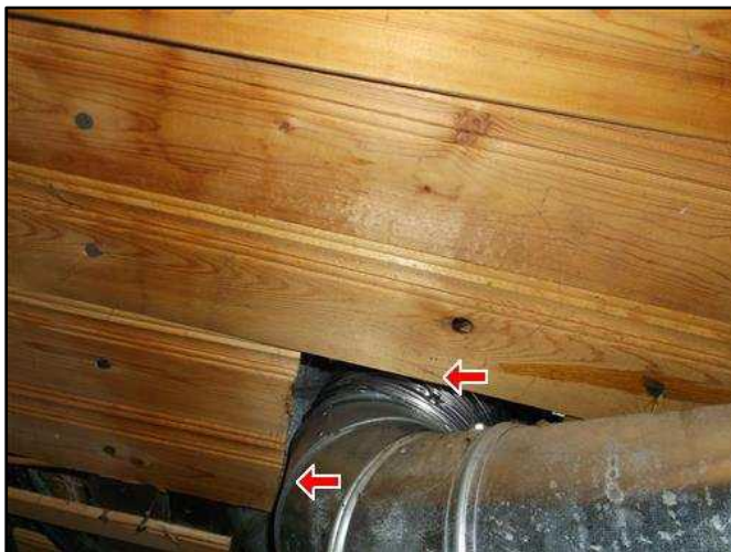
(heat system fire hazard)
