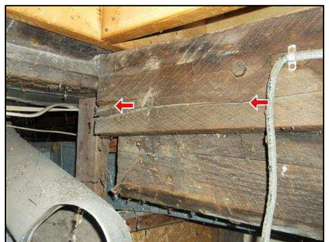
(structural basement issues)
