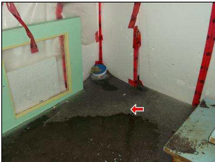
(Standing water from burst pipe in basement)
