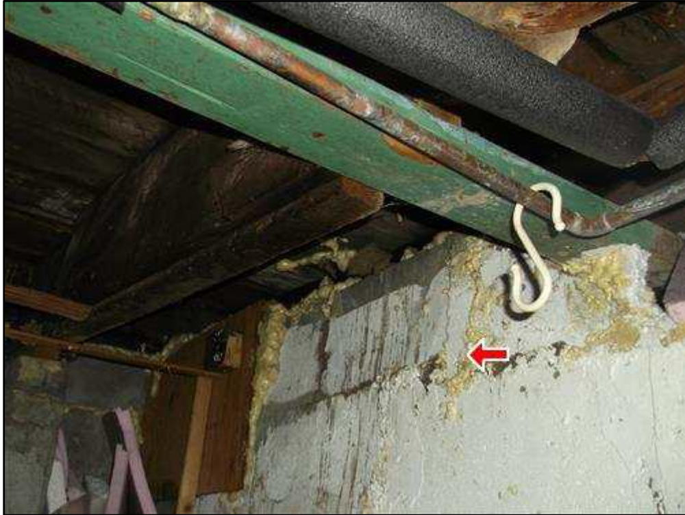
(basement foundation wall issue)
