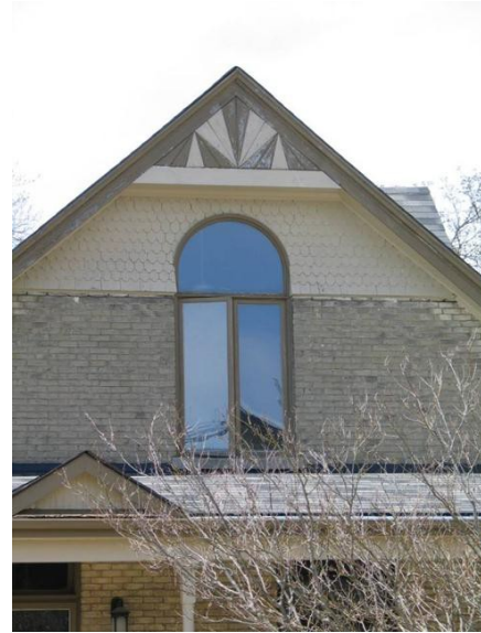
Image 19 - Window alteration, 67 Cathcart, modern intervention in sympathetic style
