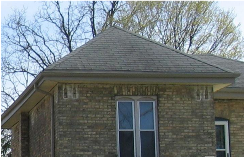
Image 34 - Missing brackets, 27 Askin
